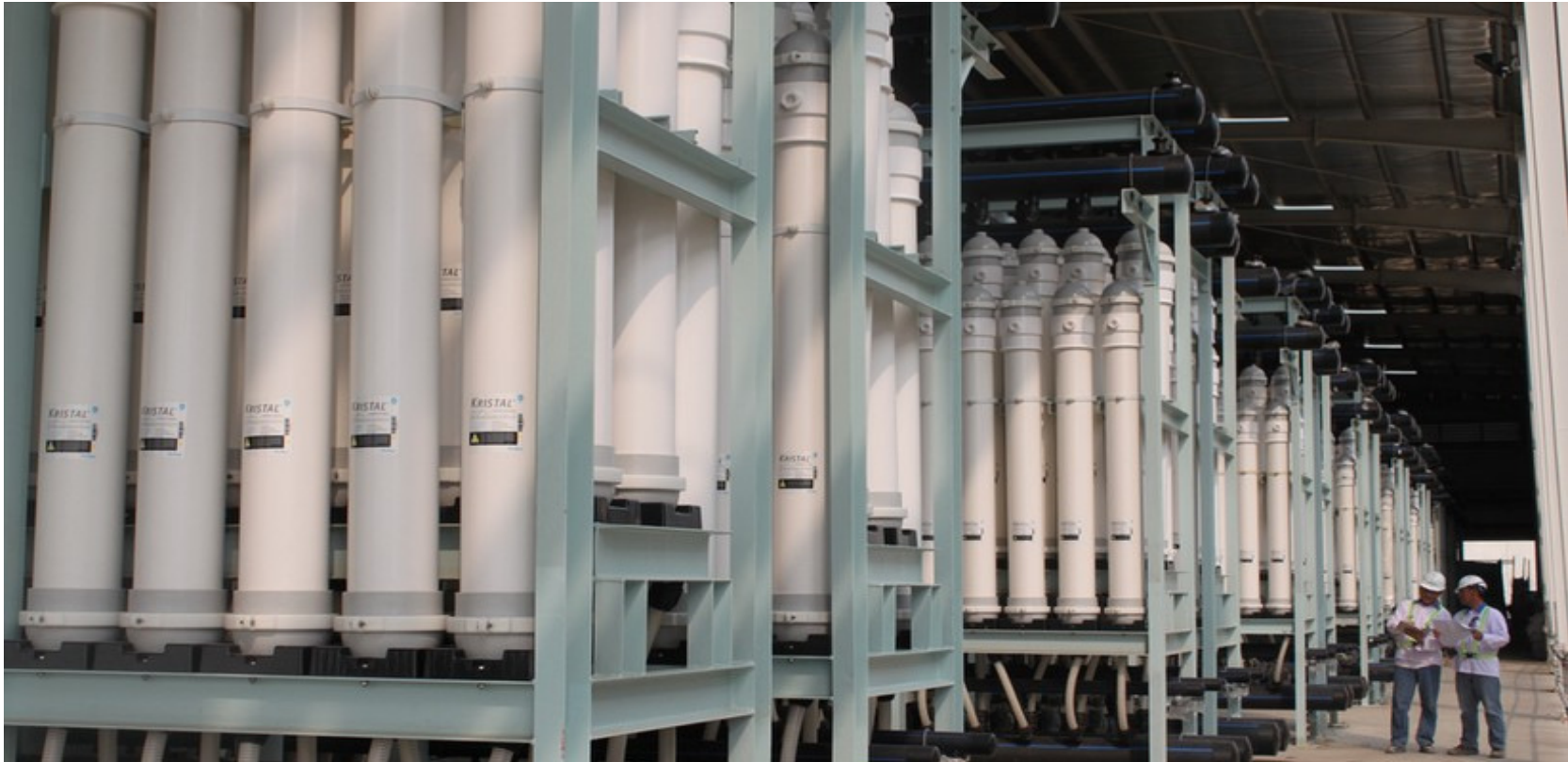
UF building housing Hyflux's Kristal ® membranes at Tuaspring Desalination Plant
